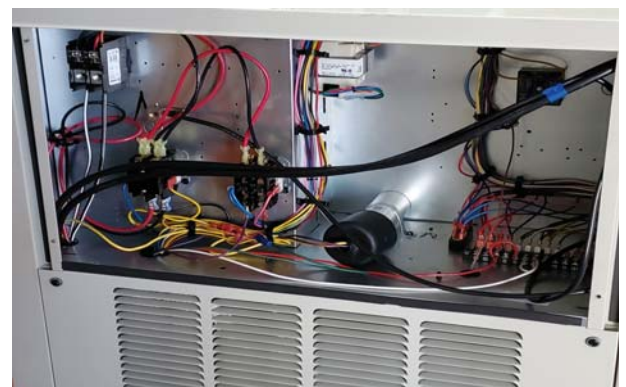
Fig. 2. Unit control compartment.
