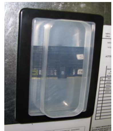
FIG. 5 - Installed breaker cover
