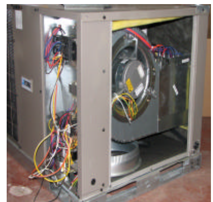
FIG. 1 – Removed control panel and blower cover.
