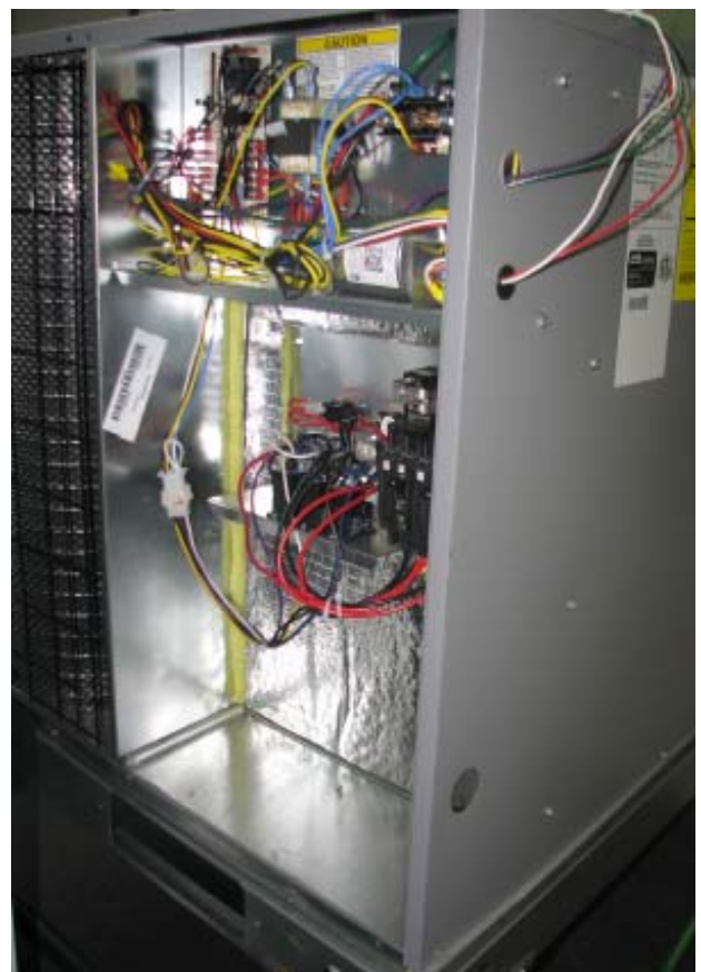
Fig. 1 - Heater access panel.
