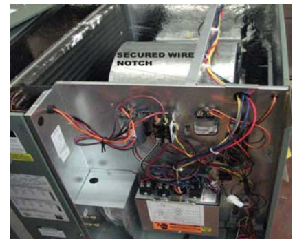
FIG. 1 - Access covers removed
