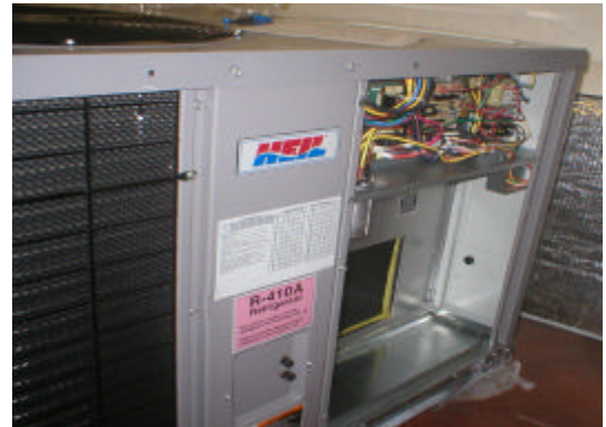
Fig. 1 - Heater access opening.
