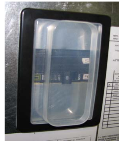
FIG. 5 - Installed breaker cover
