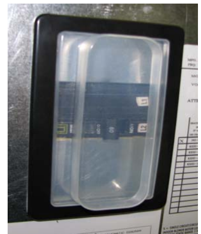
FIG. 5 - Installed breaker cover
